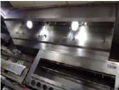
➤ Radium Kagaya hydro-vent hood
