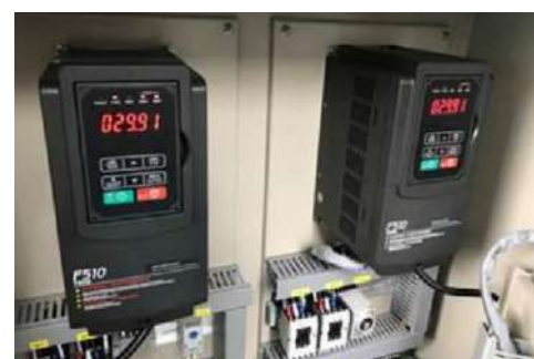
Cooling tower fan motor changed to DC inverter motor
