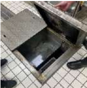
➤ Radium Kagaya grease trap
